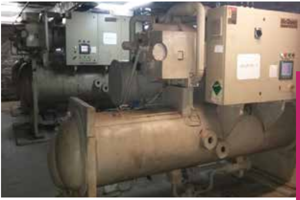
Centralized screw chiller plants at Plant-13 Annexe
