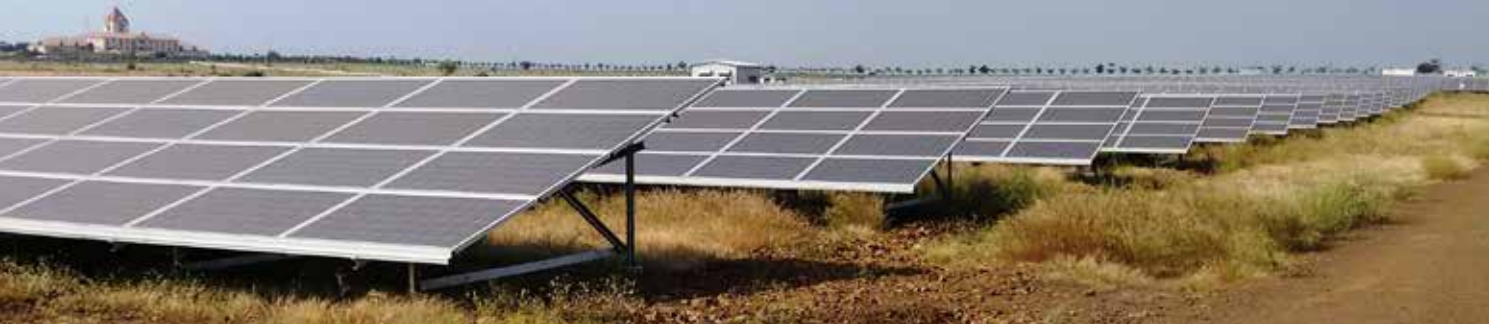
Solar PV plant under PPA
