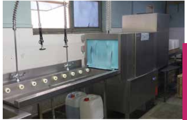
Dishwashing machine at canteen in Plant-13 Annexe
