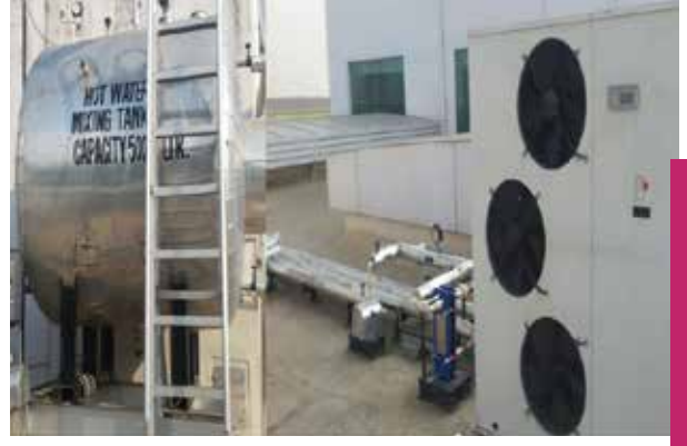
Heat pump system for hot water requirement in the kitchen at Plant-13 Annexe
